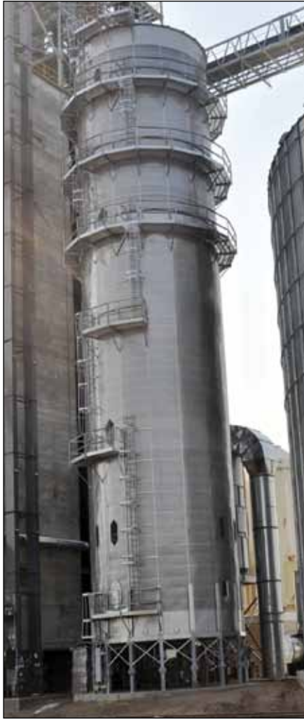
New 7,000-bph Sukup tower dryer, with Aircon baghouse dust system visible behind it.
