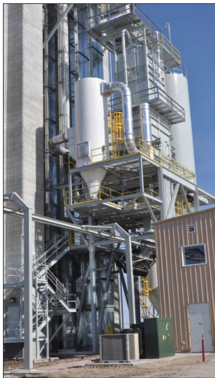
Railcar-loading site includes a 60,000-bph Intersystems bulk weigh loadout scale (top center) and a heavy-duty MAC baghouse dust collection system.
