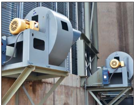
Aeration at Blanchard Valley's new tank at Fostoria is provided by four 30-hp Rolfes@Boone aeration fans.
