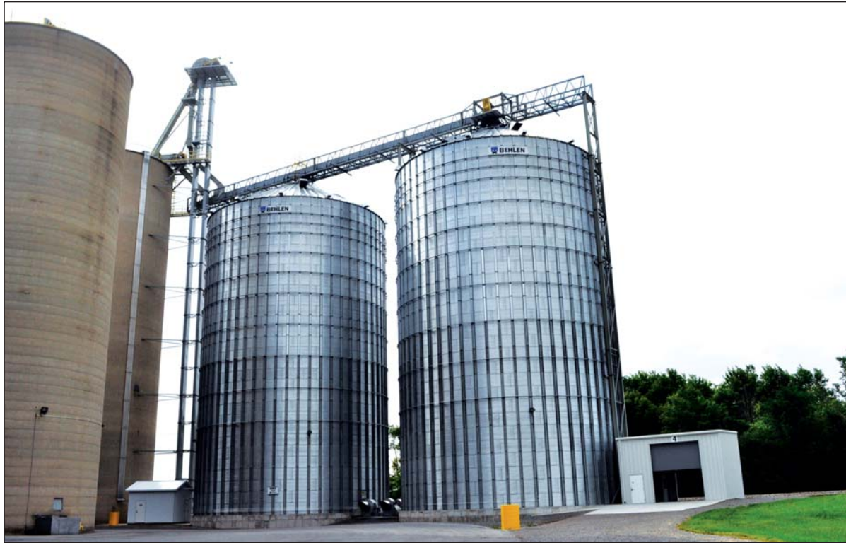
Blanchard Valley Coop upgraded its West Findlay, OH facility in 2012 with two 275,000-bushel Behlen steel tanks, a new GSI receiving leg, and a new receiving pit. Photos by Ed Zdrojewski.
