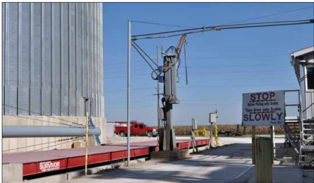
Truck scale installation at Goodland includes a new 70-foot Rice Lake pit-type inbound scale. A second Rice Lake scale is expected to be added after the 2012 harvest.
