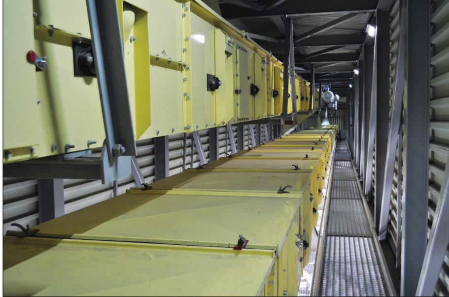
Two 1,450-tonne-per-hour Hi Roller enclosed belt conveyors carry grain out to the new storage. Ground-level photos by Ed Zdrojewski.
