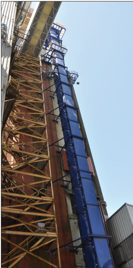
New Nordstrong 1,100-tonne-per-hour leg serves an existing cleaning house.
