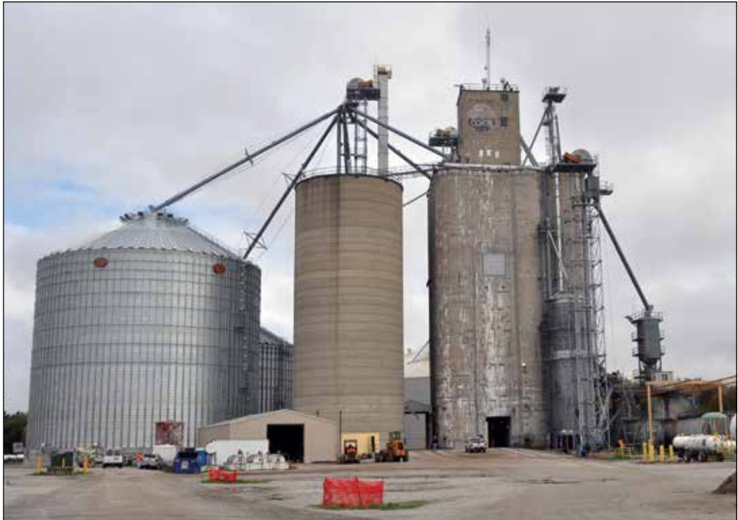
Co-Alliance, LLP's 3.1-million-bushel grain elevator at Union Mills, IN, a little over a year after an explosion damaged portions of the concrete workhouse and adjacent grain dryer. The 700,000-bushel GSI steel tank at left is new. Photos by Ed Zdrojewski.
