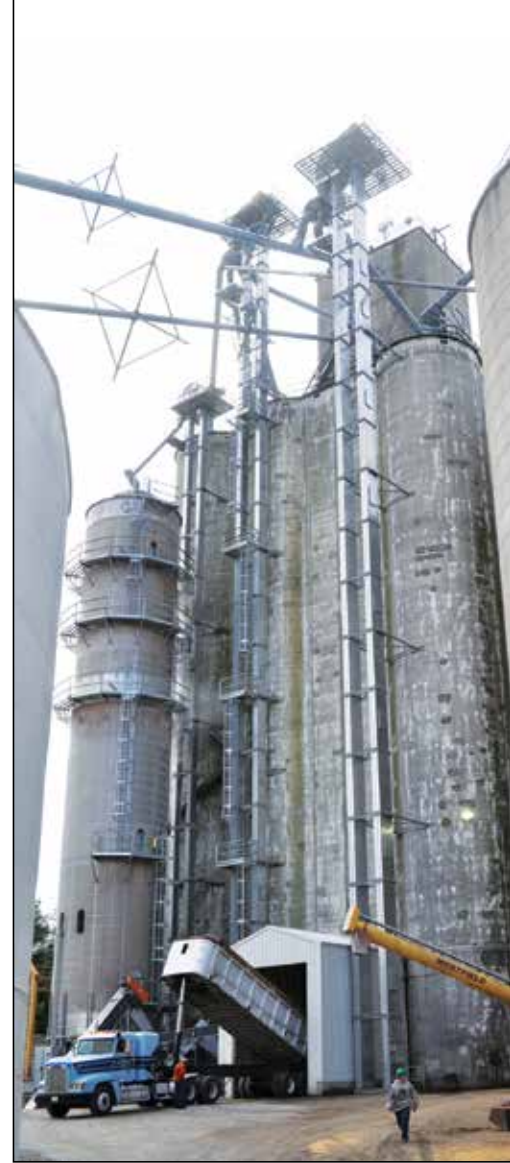
Producer deposits a load of grain into a new receiving pit, which feeds a new 25,000-bph GSI outside leg at right.
