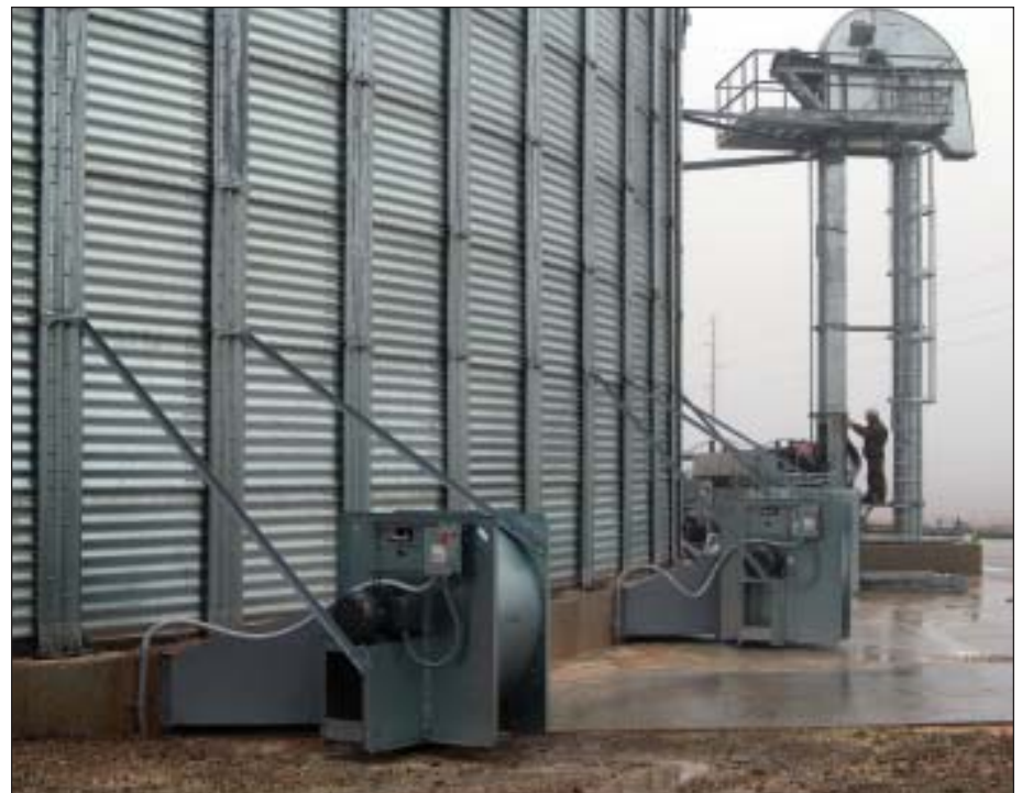
Workers in November 2008 put the finishing touches on a 15,000-bph Chief jump leg serving a 1.1-million-bushel Chief Titan steel tank. The tank is already filled with dry corn.
