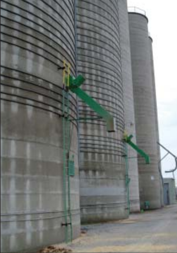
Side draws were moved to the west side of the existing tanks to reconfigure the traffic flow at the elevator.
