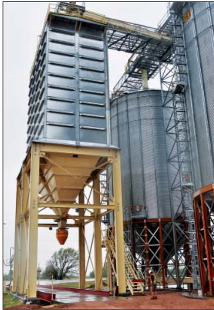
An InterSystems' square bolted bin equipped with a Sioux Steel dust suppression hopper and spout loads trucks atop a 120-foot outbound Fairbanks truck scale.
