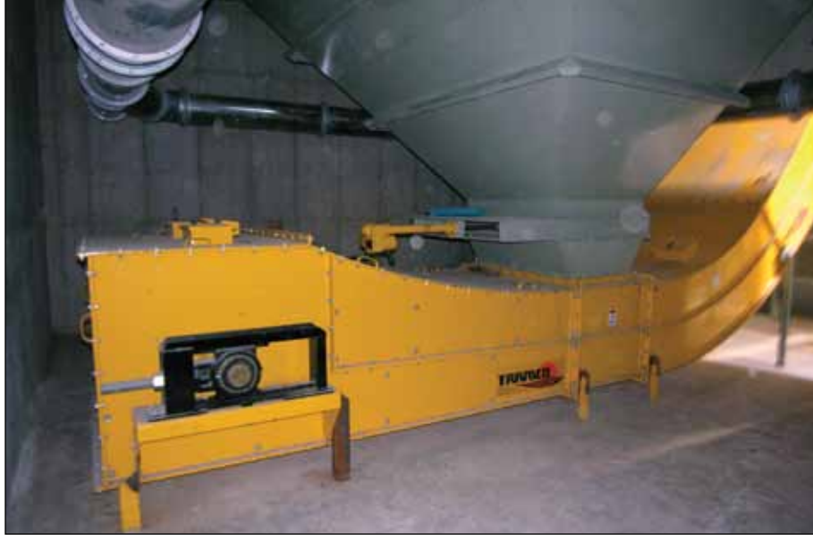
Facility's third receiving pit empties onto a 30,000-bph Tramco drag conveyor that inclines up to a GSI receiving leg.
