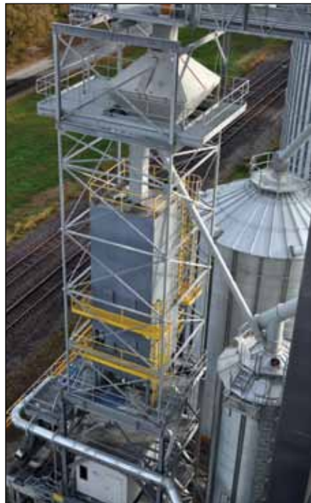
Overhead view of a 40,000-bph Intersystems gravity screener and 40,000-bph Compu-Weigh bulk weigh loadout scale.
