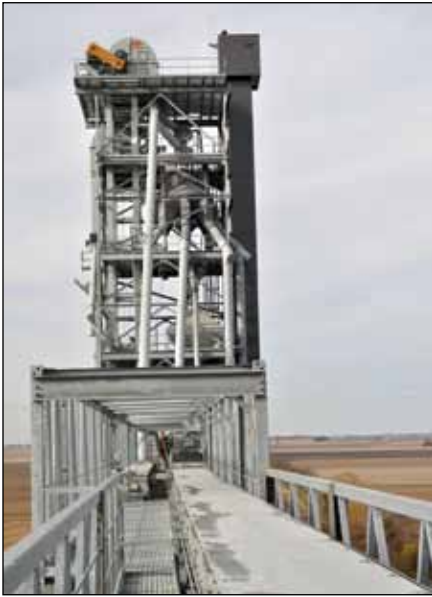
Rooftop equipment visible includes a 20,000-bph, head sections of three GSI legs, top section of a PMI (Schumacher) 650-lb.-capacity manlift, eight-hole Union Iron Works double distributor, and 20,000-bph Intersystems gravity screener.
