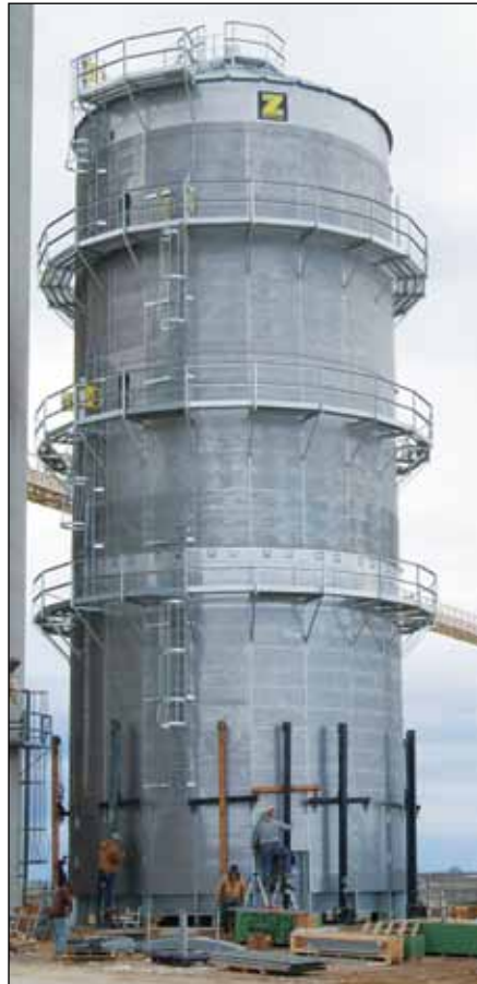
New 10,000-bph Zimmerman tower dryer under construction at Madison early in May 2011.
