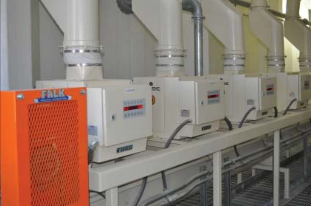
A series of eight Buhler flow controllers route product through the complex flow required for the large variety of animal feeds produced at Casa Grande.
